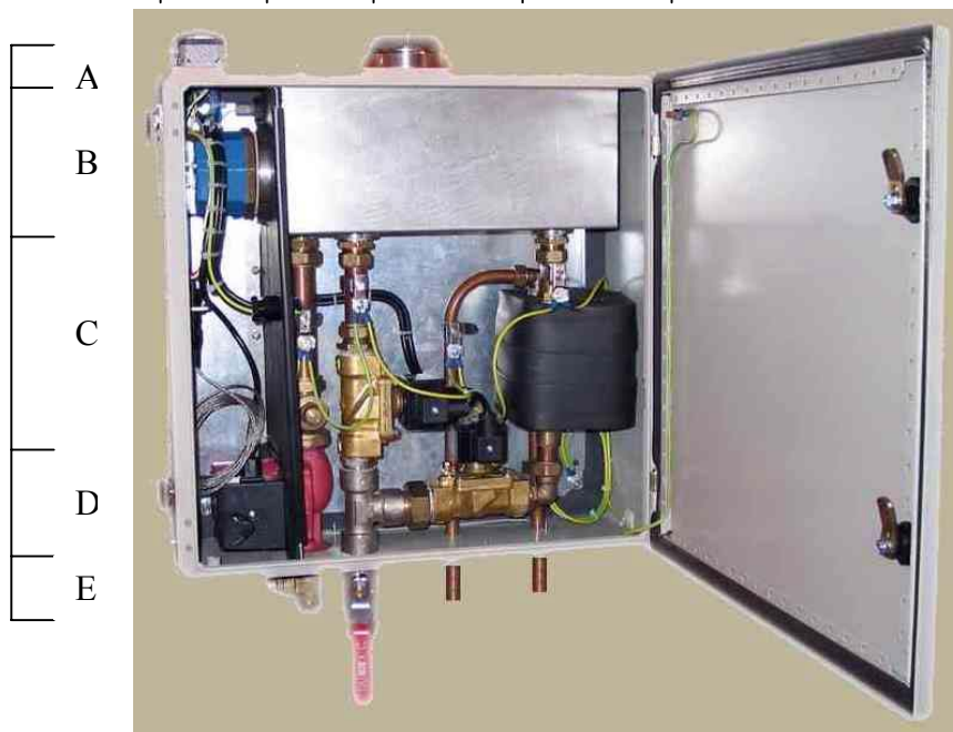
Fuel Condi tioning Unit (FCU) : Stainless Header Tank (B3/4) Fill Cap (A3), Heat Exchanger in black insulation (C4), Selector Valves (C2&D3), Immersion Heater (B1), Circulation Pump (D2) Process Water Lines (E2), Chilled Water Lines (E3/4), Electrical Connector (A1).
